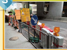
竹園道近竹園北邨 Chuk Yuen Road near Chuk Yuen North Estate
